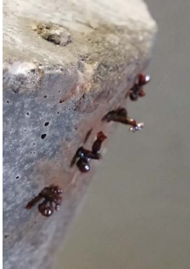
Figure 4.25 Carbon steel wires protruding from sample P2 Photograph by Dietrich Vogel copyright 2016 by Dietrich Vogel
