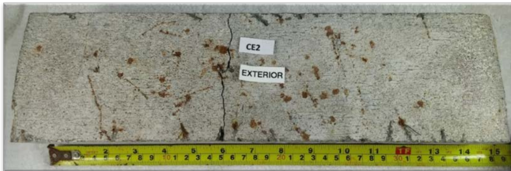
Figure 2.10 Beam sample CE2; modulus of rupture 910 PSI Photograph by Dietrich Vogel copyright 2016 by Dietrich Vogel
